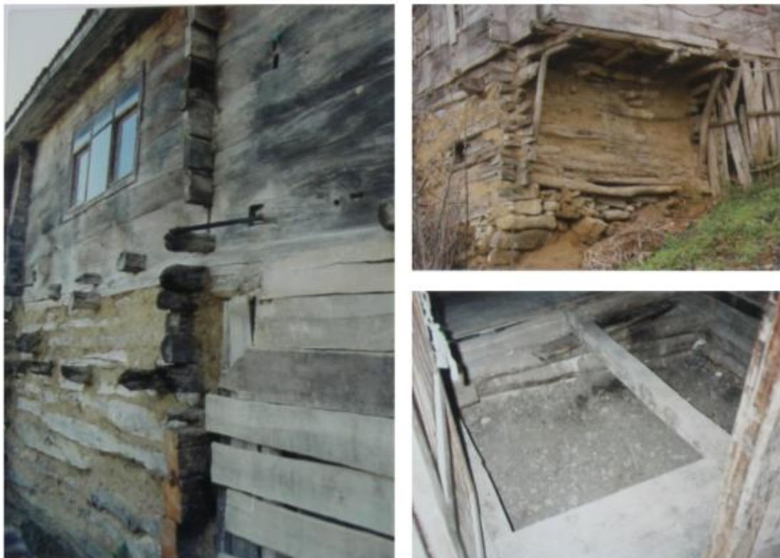
Photo 6. The isolation gap between the barn and the living space in two-storey traditional houses.
